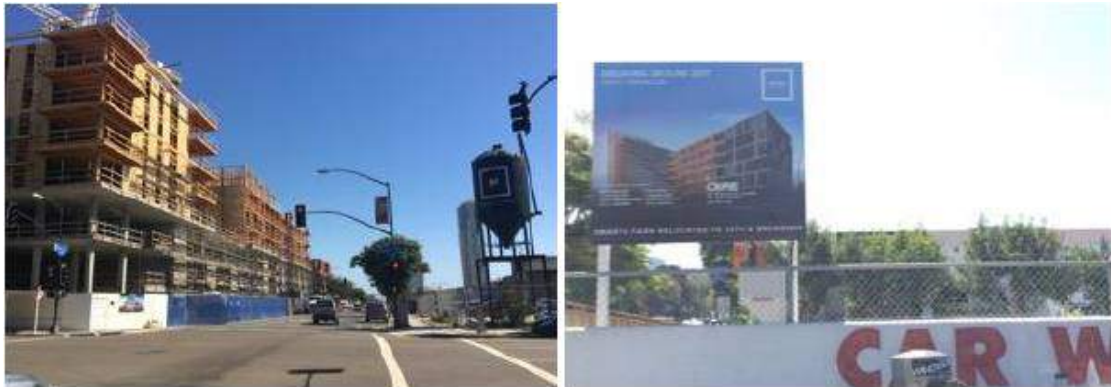
Figure 20 - Makers Quarter Construction Site. (Source: Authors' pictures) (Figure 17 in Annex 1i – Laura Biancuzzo, Luana Parisi)
